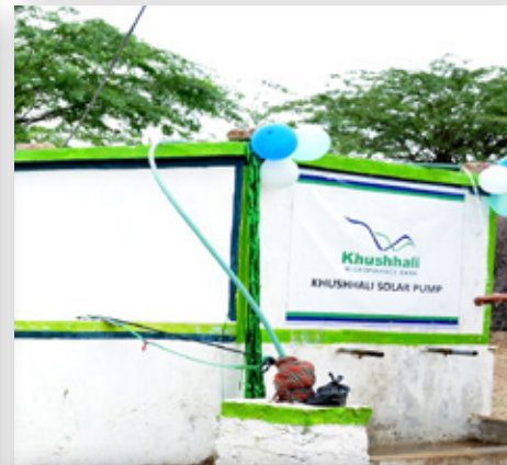
SOLAR POWERED DRINKING WATER FACILITY, THARPARKAR
