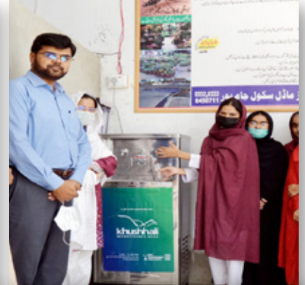
DRINKING WATER COOLERS WITH FILTERS INSTALLED IN GOVERNMENT SCHOOLS OF DG KHAN
